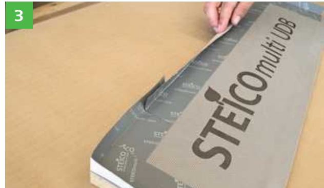
3 The STEICOmulti tape F adhesive strips are then attached to the insulation wedge in such a way that a three-sided „trough“ is formed.
