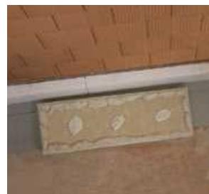
Adhesion of insulation boards on uneven surfaces using the point and bead method
