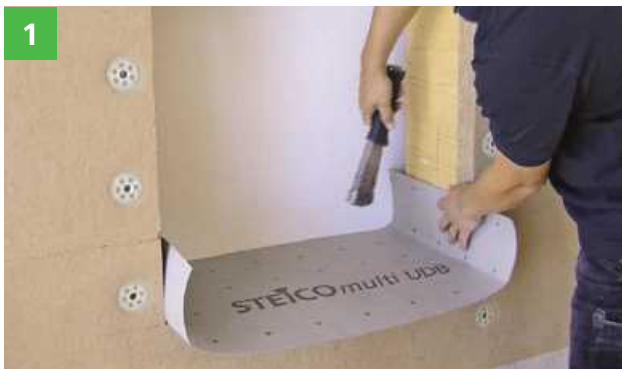
1 Attachment of STEICOmulti UDB (diffusion-open membrane) as temporary weather protection until window installation.
