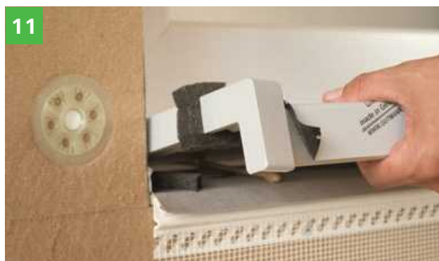
Installation of windowsill. TIP: The rear sheet metal interlocking is located in the matching window groove, the front one has a distance of \geq 3 cm to the render facade TIP: Storing Compriband strips in the cool box prevents them from expanding too quickly.
