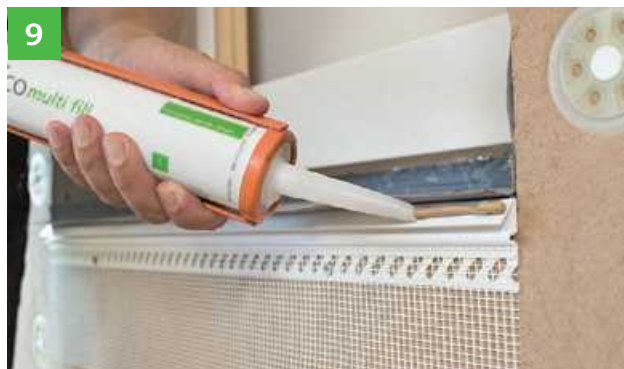
The protruding flap of the laminated underlay is glued to the drip edge of the parapet profile using STEICO multi fill .
