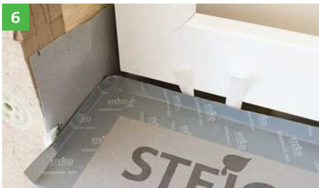
Installation of the STEICO fix insulation wedge. TIP: Fold back release paper, it can be removed more easily later.
